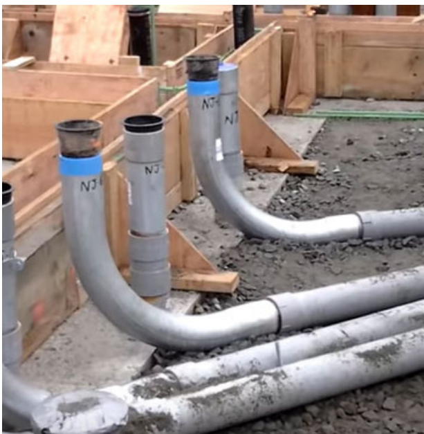
PVC Conduit Stubbed-Up with GRS Elbows
